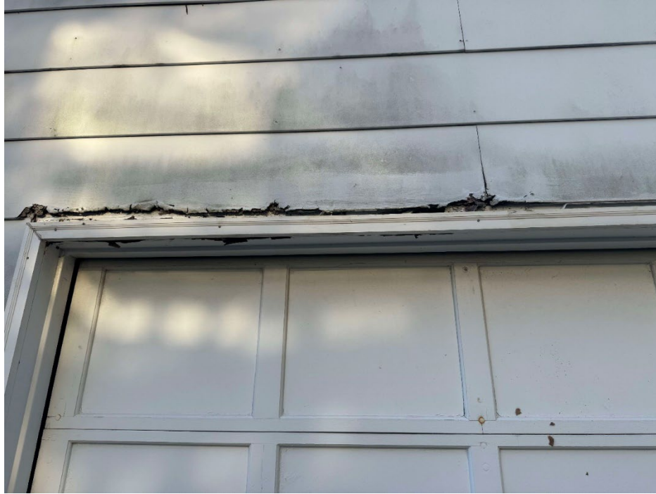
106 North 6 th Street | Closeup of deterioration on siding above garage door | 8/2025 (applicant)
