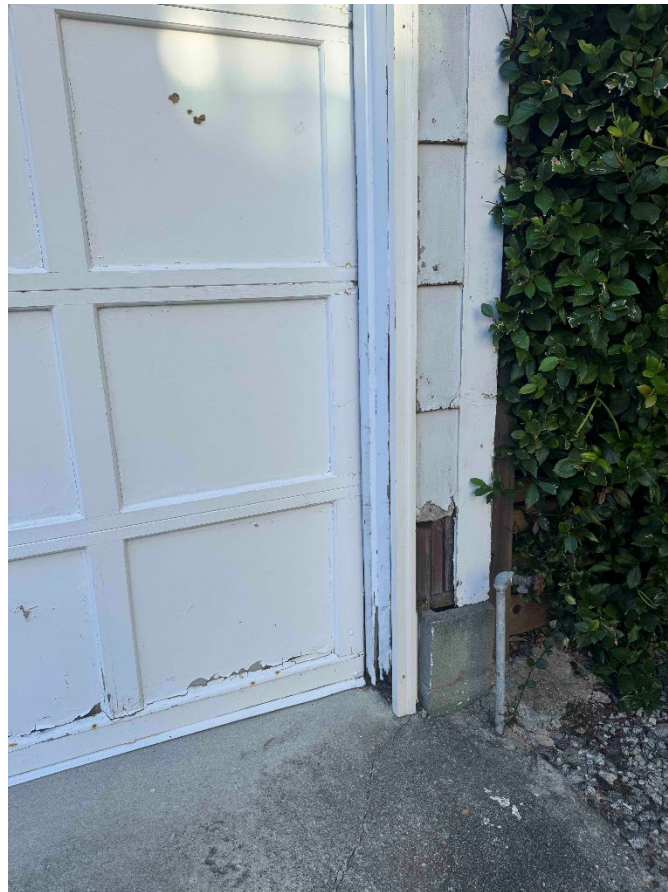
106 North 6 th Street | Closeup of deterioration on garage door and siding | 8/2025 (applicant)
