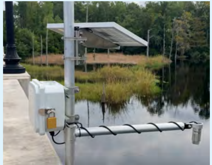
The flood gauge on the Love Grove Bridge, installed at the confluence of Smith Creek and Burnt Mill Creek, is one of seven locations where water levels are being monitored in the city.
