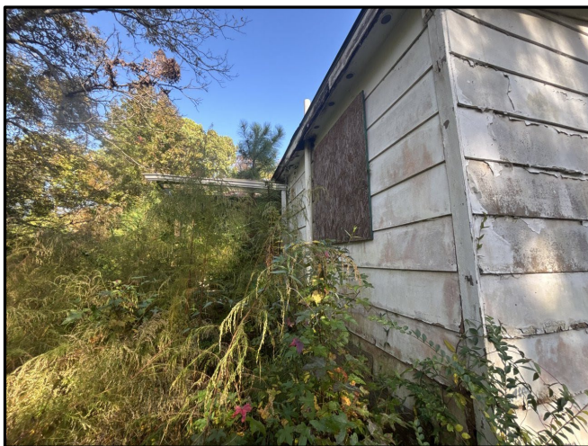
The west side of the residential structure on Tract 3; Picturing a vent pipe typically used for plumbing purposes.
